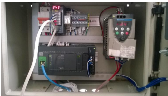
Fig. 7. Layout Inside Electrical Control Box.
