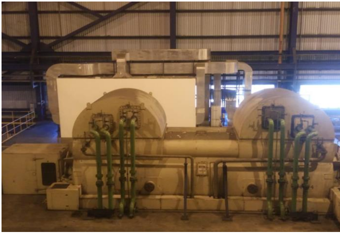
Fig. 3. Generator in a Steam Power Plant.
