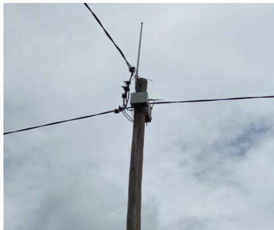
Fig. 4. LoRa Base Station Installed at the Pole.
