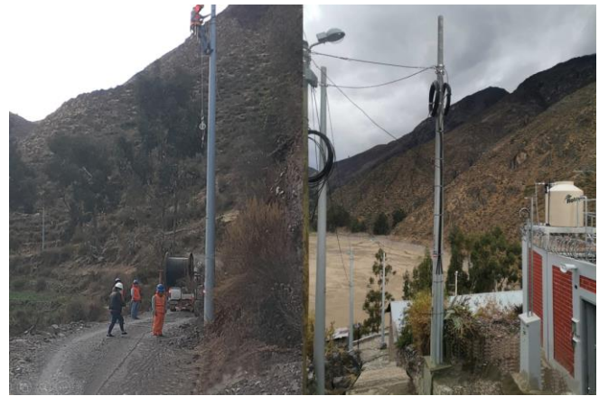
Fig. 7. Optical Fiber Installed in the Lima-Peru Region.
