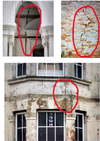
Fig. 1. Condition from the front side of the cracks of several ancient buildings in the old town of Semarang
