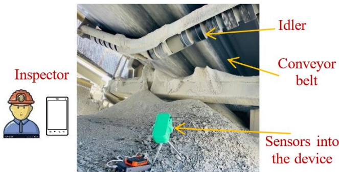
Fig. 1. The prototype installed in “MMG Las Bambas” mining company (Peru).
