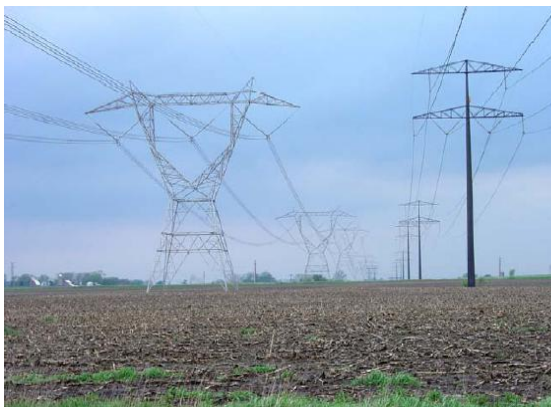
Fig.1. a. Lattice (left) and Monopole (right) Towers (Source: Argonne Staff Photo)
