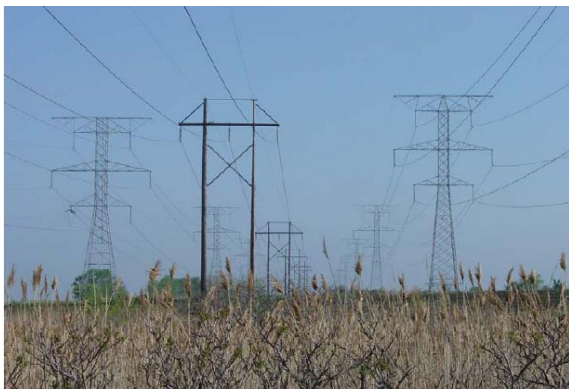
Fig.1. b: Multiple lines in a power Corridor (Source: Argonne Staff Photo)
