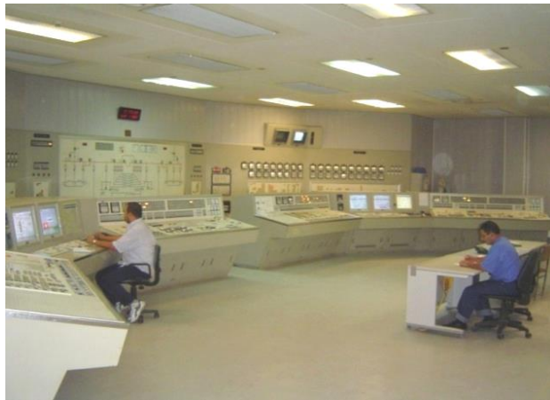
Fig. 3. Control room of the TPP
