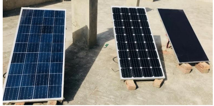
Fig. 1. PV Modules Installed at Experimentation Site.
