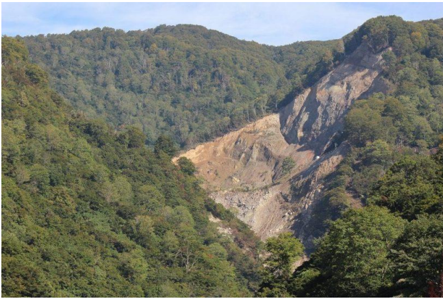
Fig. 6. Photograph of the slope failure area.
