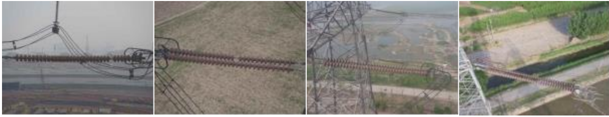
Fig. 1. Image of partial insulator defects.
